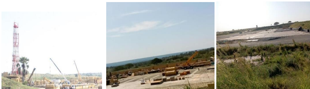
Figure 5: Activity variation at JBR4- Drilling, rig demobilization and post drilling activities e.g., site cleaning at JBR4
