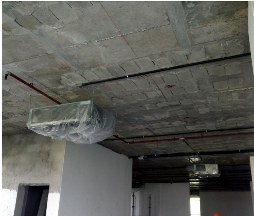
Fig 89; In door AC machines fixed onto slab soffits.
