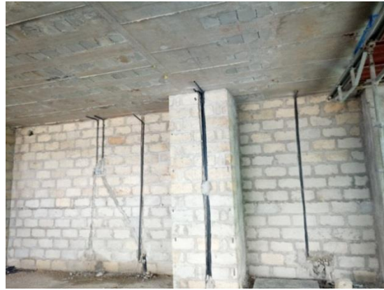
Fig 59; Conduits and mks fixed to wall.
