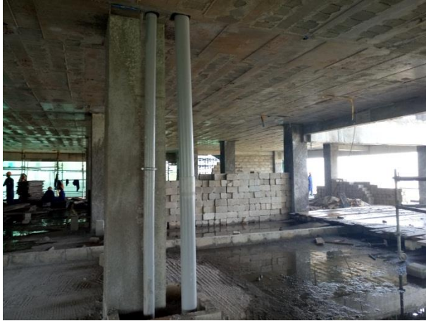
Fig 53; PVC pipes for rain water from roof.
