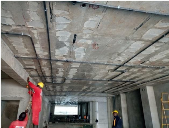
Fig 58; BMS conduits fixed to slab soffit.
