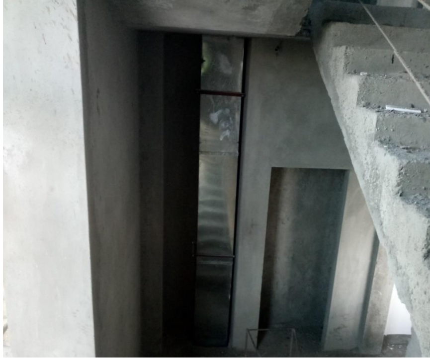
Fig 88; Pressurization ducts fixed along staircases.
