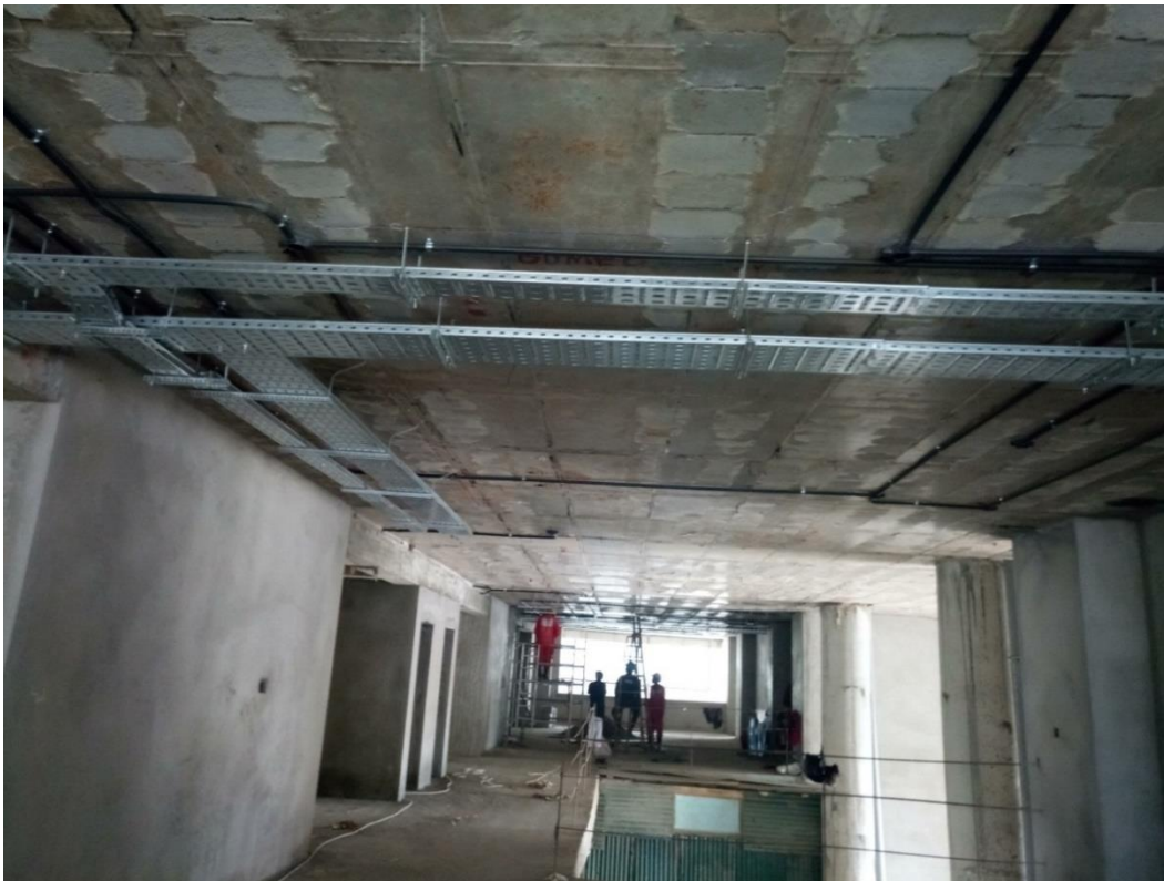
Fig 60; Cable trays fixed onto slab soffits.
