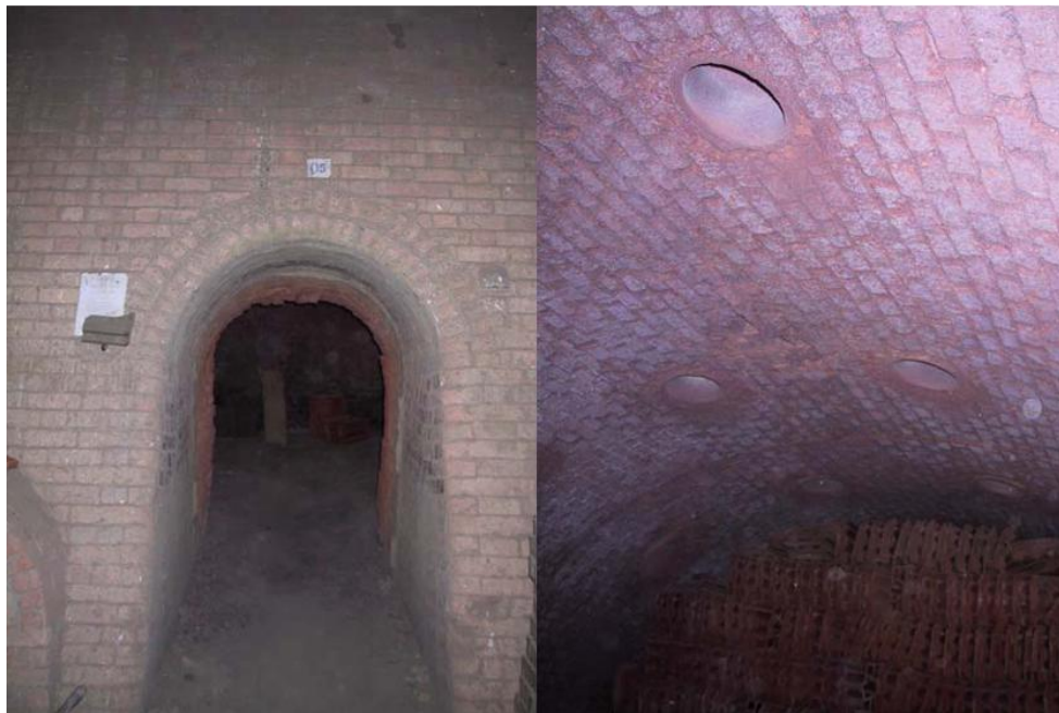
Figure 2.6: Hoffmann kiln at Uganda Clays with holes in the ceiling of the kiln used to feed coffee husks into the kiln (Source; Bingh, 2004)
