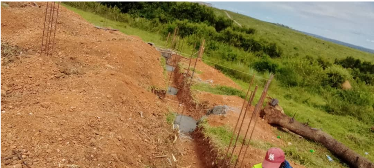
Photograph showing column footing of the one unit three classroom block facility
