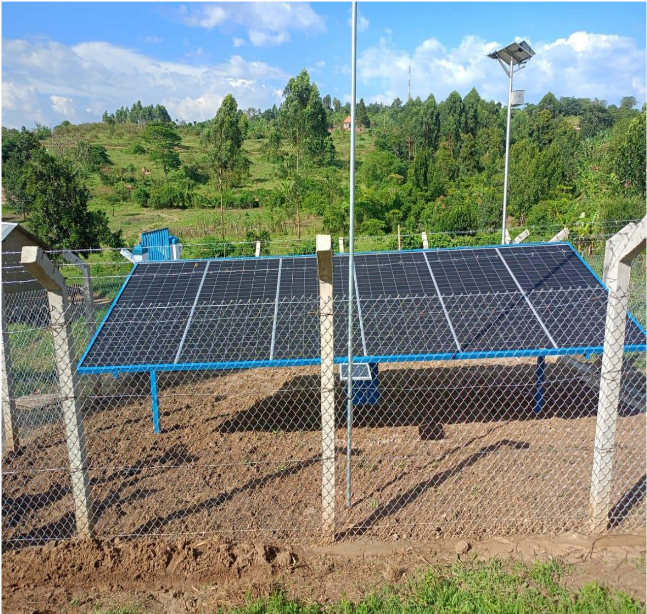
Solar panels installed on the borehole.
