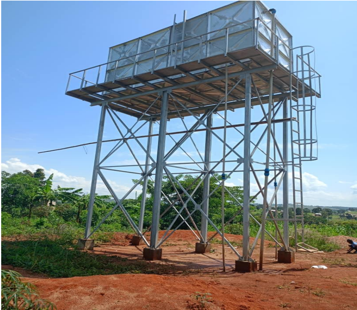
Raised Reservoir tank of 32,000l
