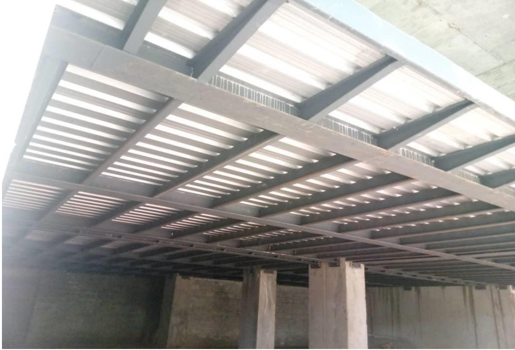
Figure A 8. A photo showing the soffit of an SSD slab.
