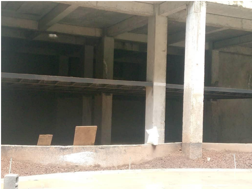
Figure A 11. A photo showing the position of an SSD slab as an intermediate/mezzanine slab
