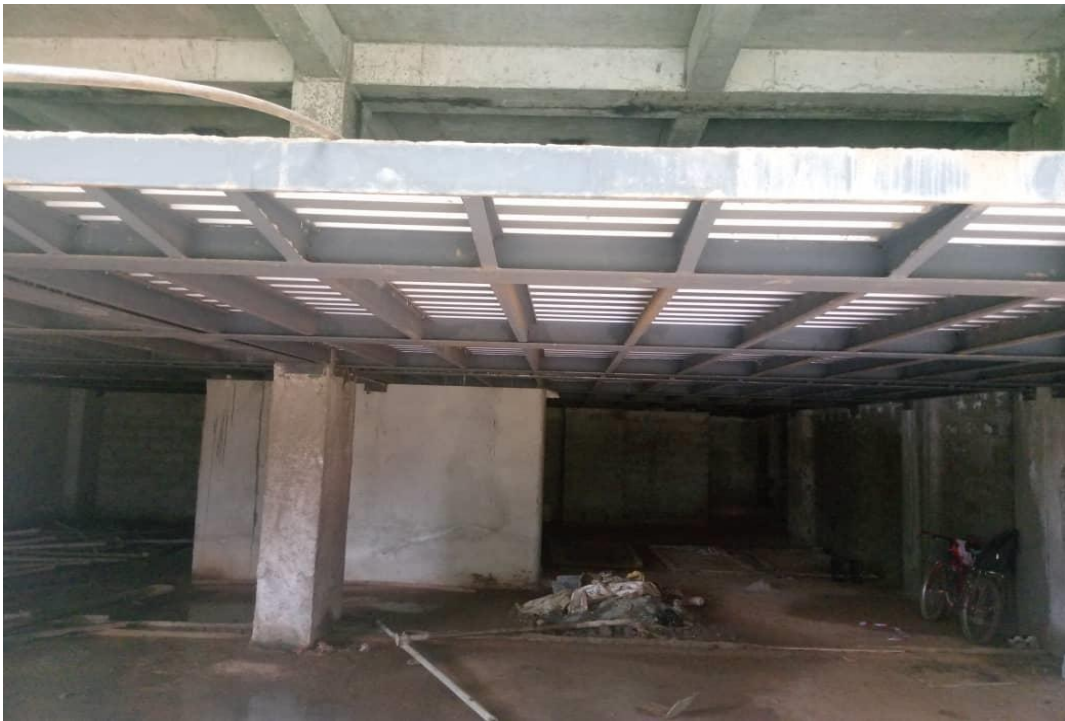
Figure A 9. A photo showing the integration of an SSD slab within an RCC framed structure
