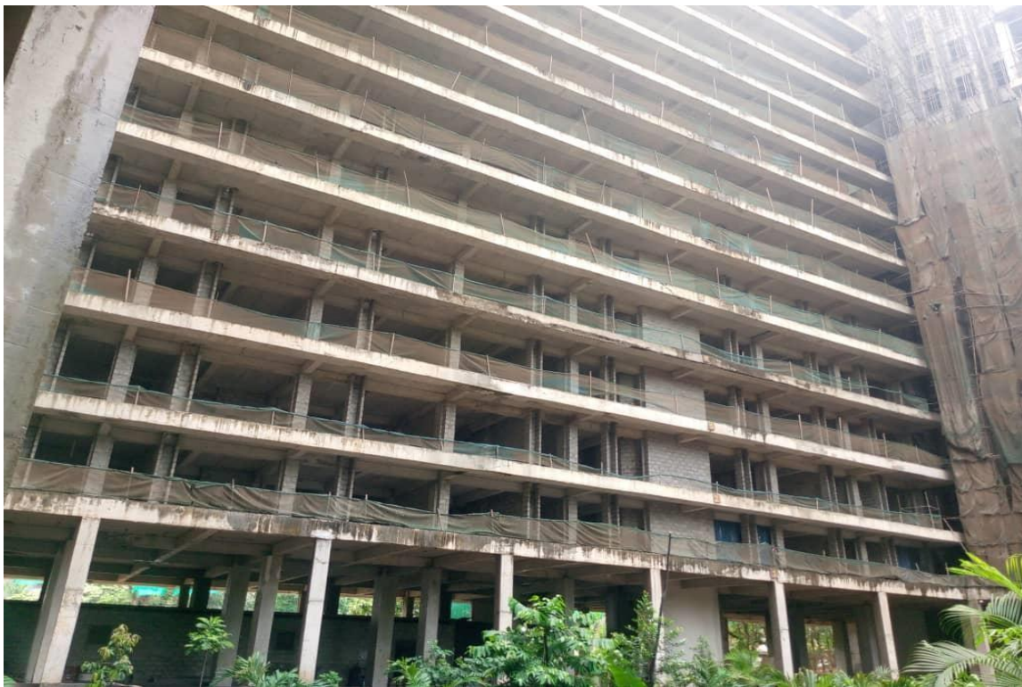
Figure A 7. A photo showing the different floor/levels on BLOCK B of the project
