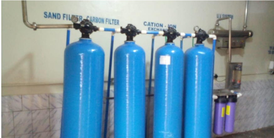
Photo 1: A water treatment system used for treating process water in a Kombucha processing plant in Wakiso, Uganda
